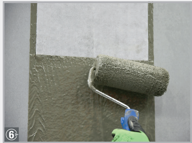
Apply the second coating layer. Layer thickness: approximately 1.2 mm Usage: approximately 0.6 kg per metre/joint The edge area of the non-woven must be completely covered.
